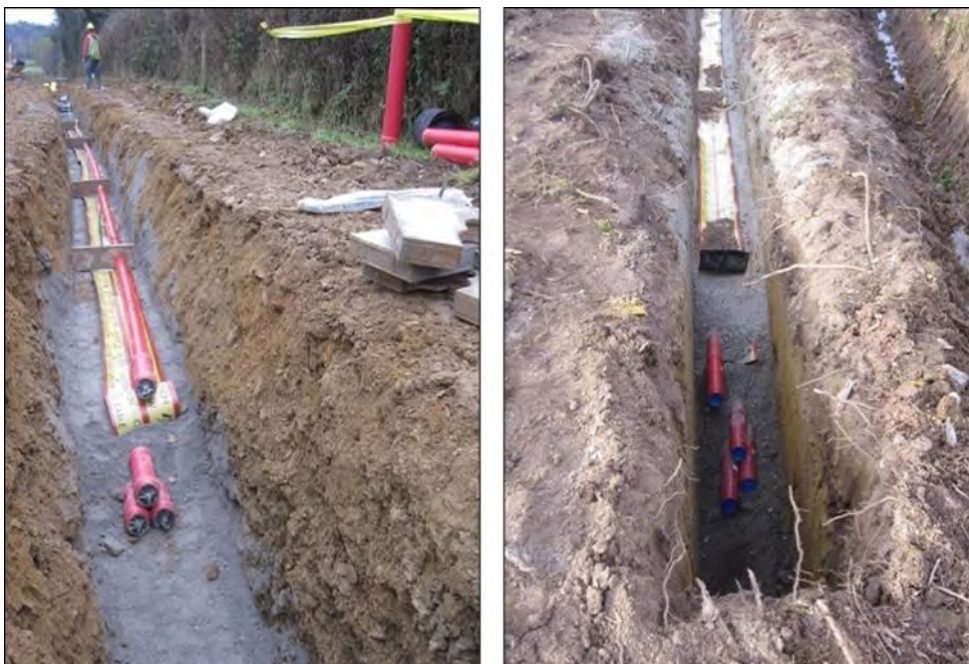
Plate 4-9 Typical Cable Trench View
